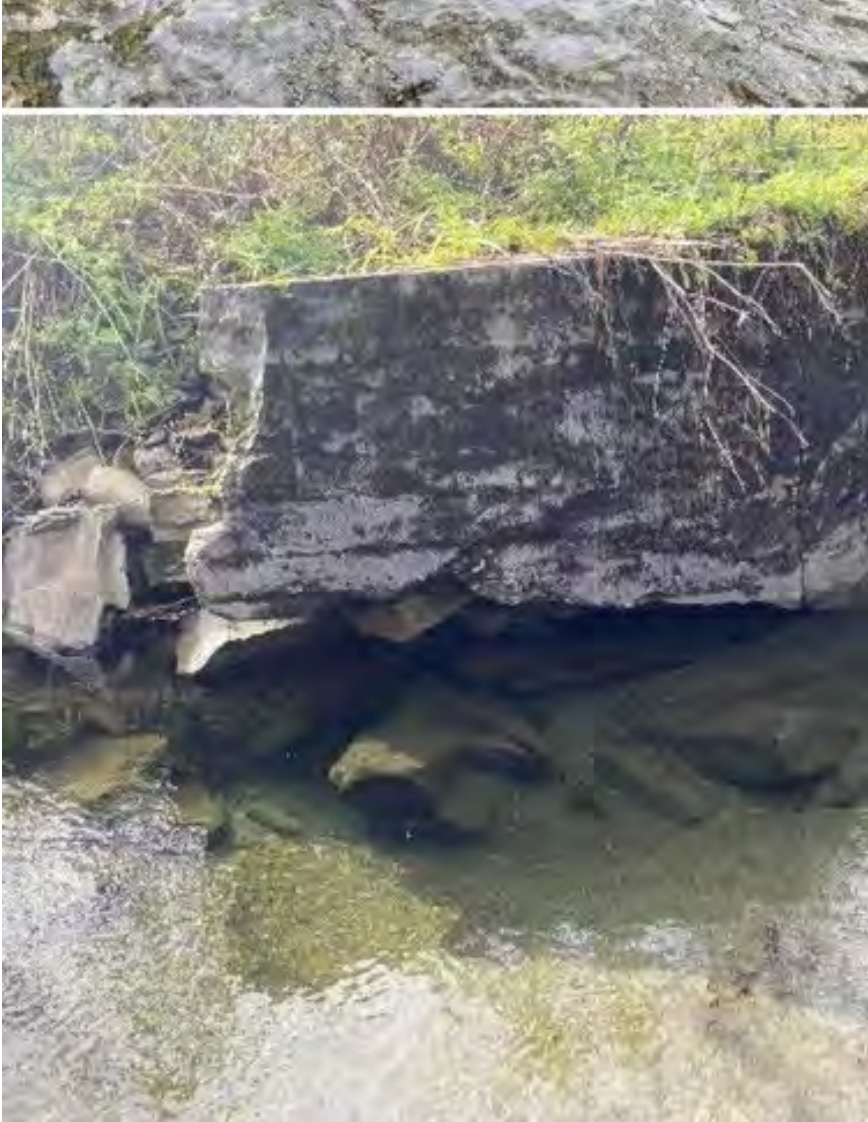
View of the undercut abutment
