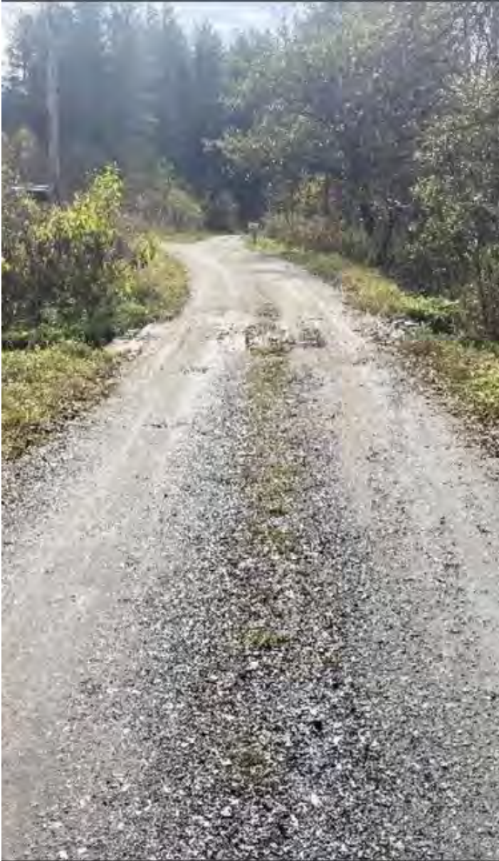
The July 2023 FEMA storm event overtopped the road and washed out half the road due to undersized structure
