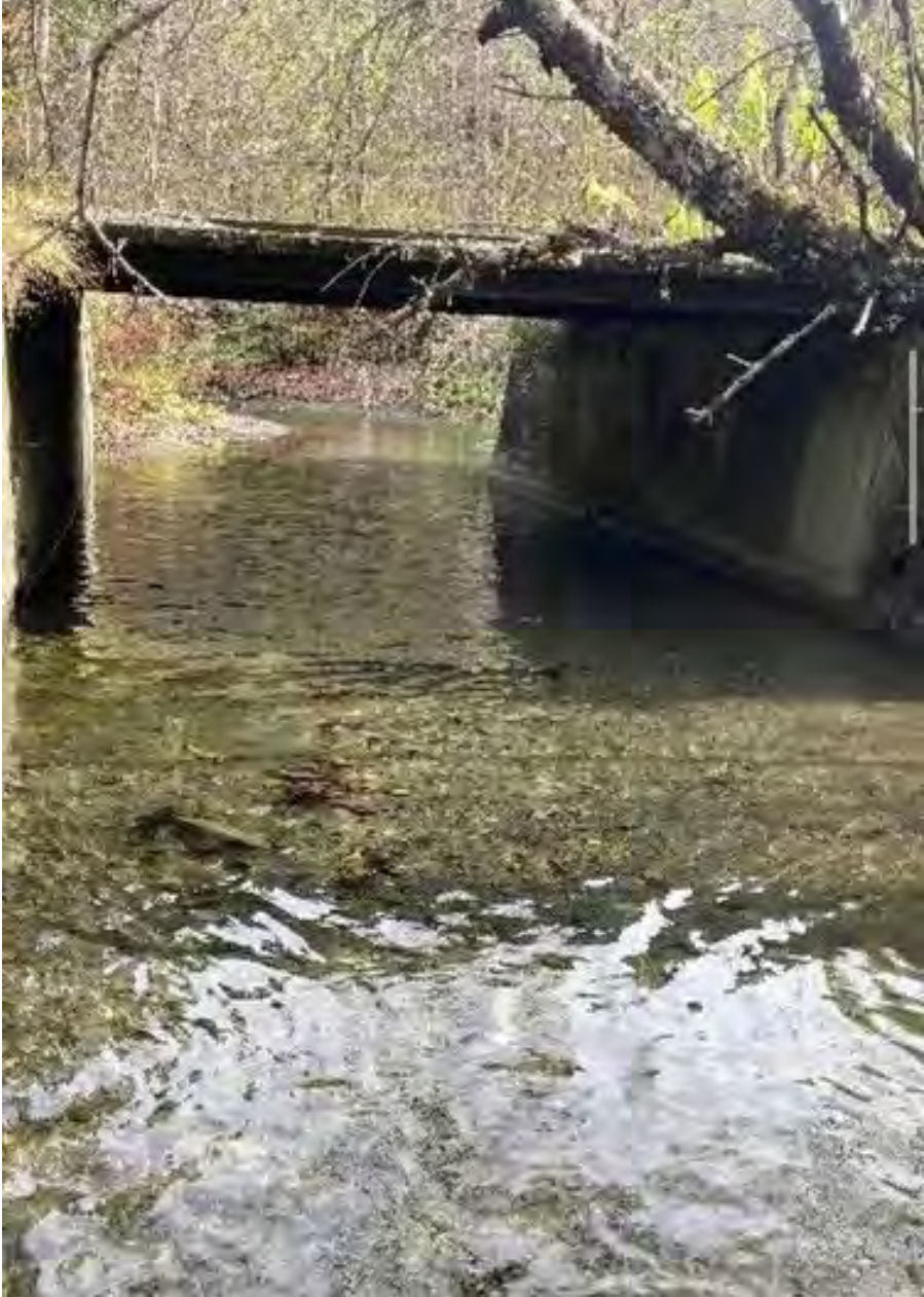
View of the undersized opening of the bridge
